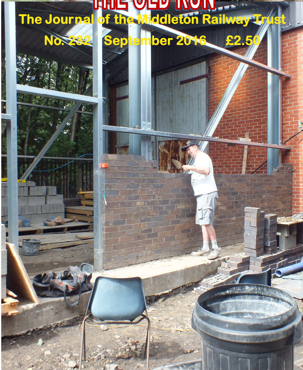
A brilliant Brickie, Andy, at work on the Running Shed. Come and view our progress!
