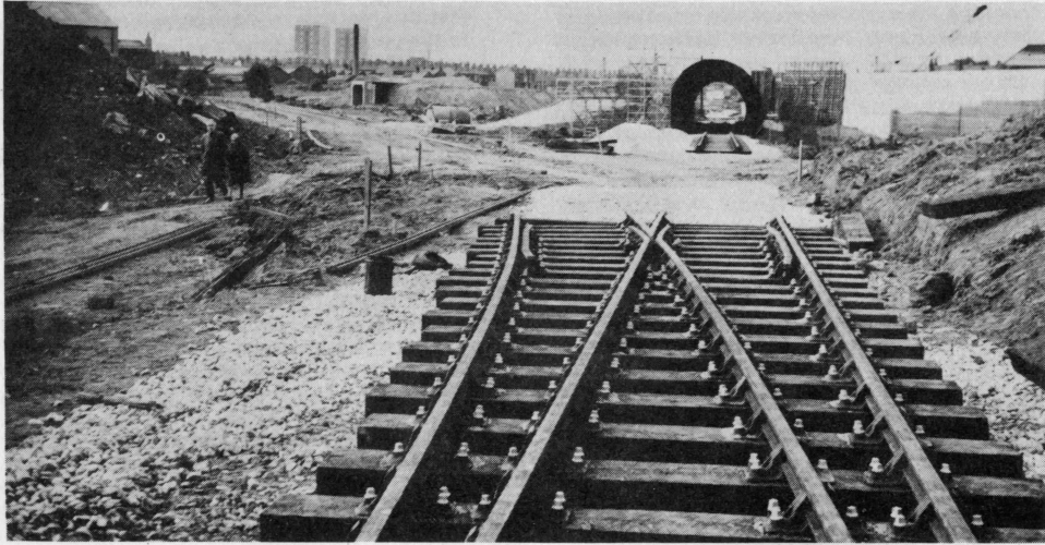
Construction — a view along the earthworks of the new line to Dartmouth works, before tracklaying commenced.
