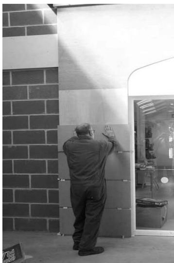
On 3 June 2006, Dave Cook is busy constructing the replica Kitson Locomotive Works arch inside the Engine House (Andrew Johnson)
