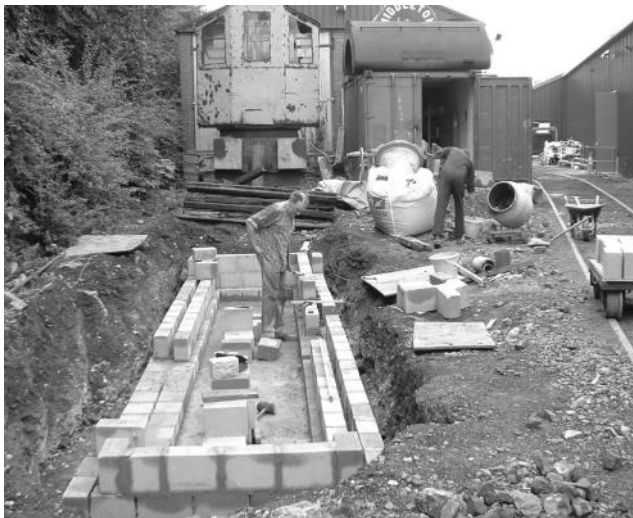
The locomotive servicing pit is well underway on the line of track leading to the Old Shed, where ultimately the running shed is to be built, 22 July 2006 (Andrew Gill)
