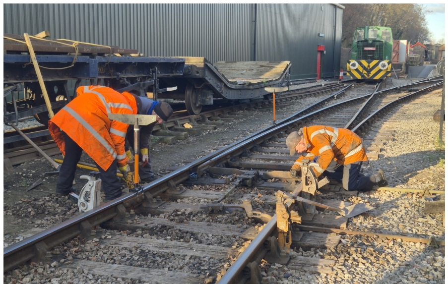
Trackwork in progress on 3rd January on the Moor Road Yard turnout.
